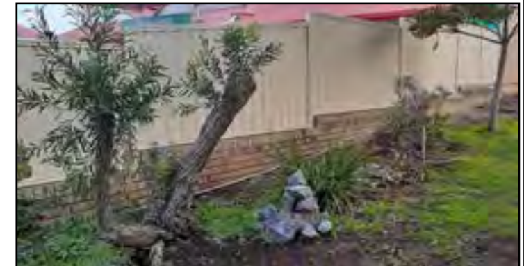
New shared fence between petrol station and church is most welcome to the Community Garden
