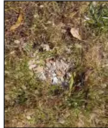
Hydrant cover with poor access
